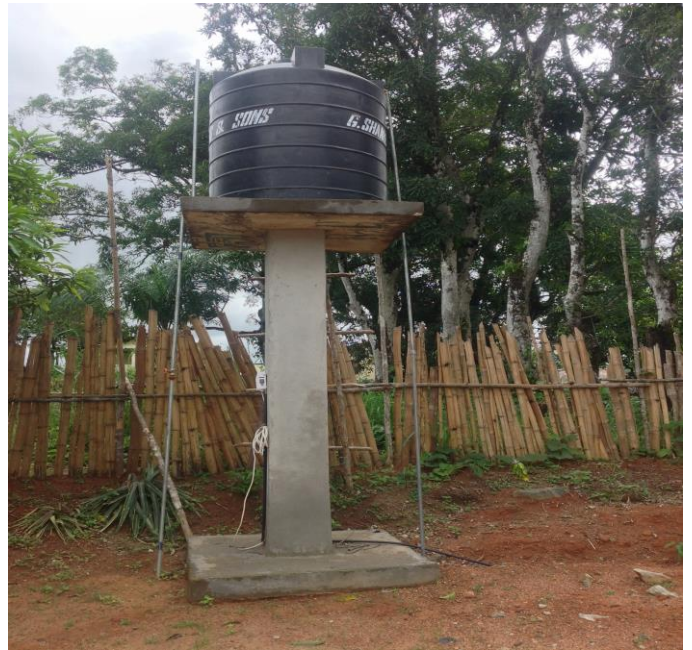
water tank that feeds directly to facet next to the clinic
