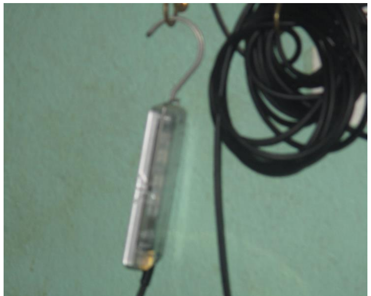
extension cord that leads to outlets
