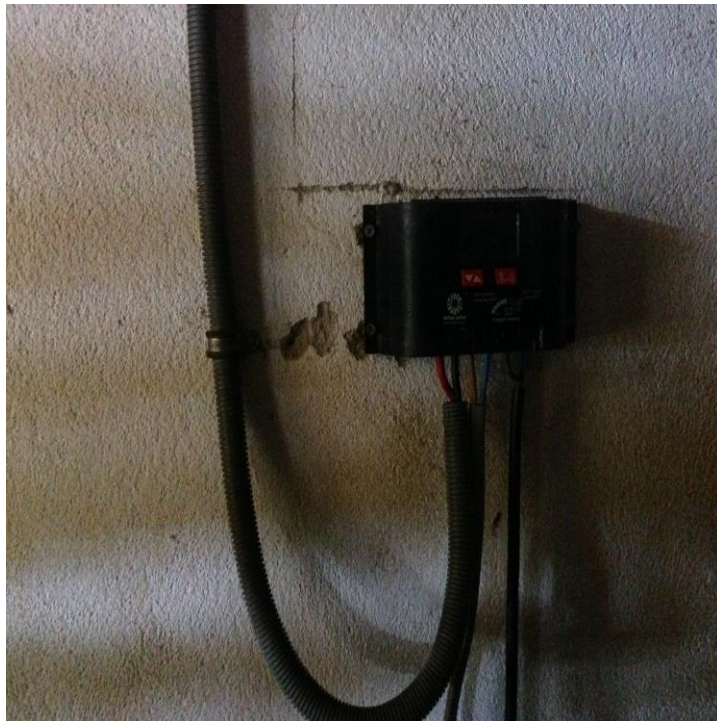
Additional solar wiring inside
