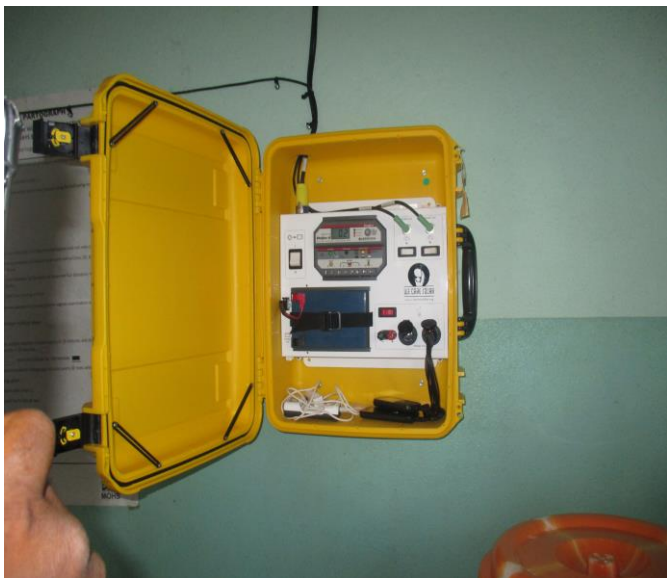
solar control panel inside the health clinic
