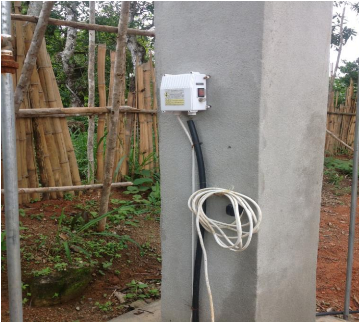
Pump and energy wiring
