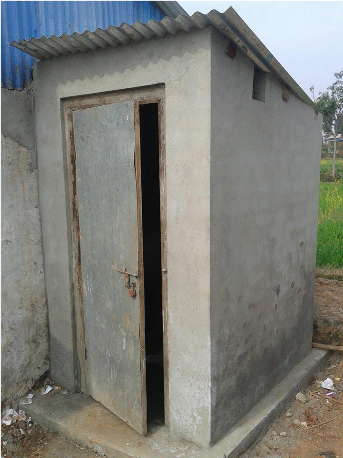
This newly constructed toilet was built to replace a toilet destroyed at the school in Deuralitar Village.
