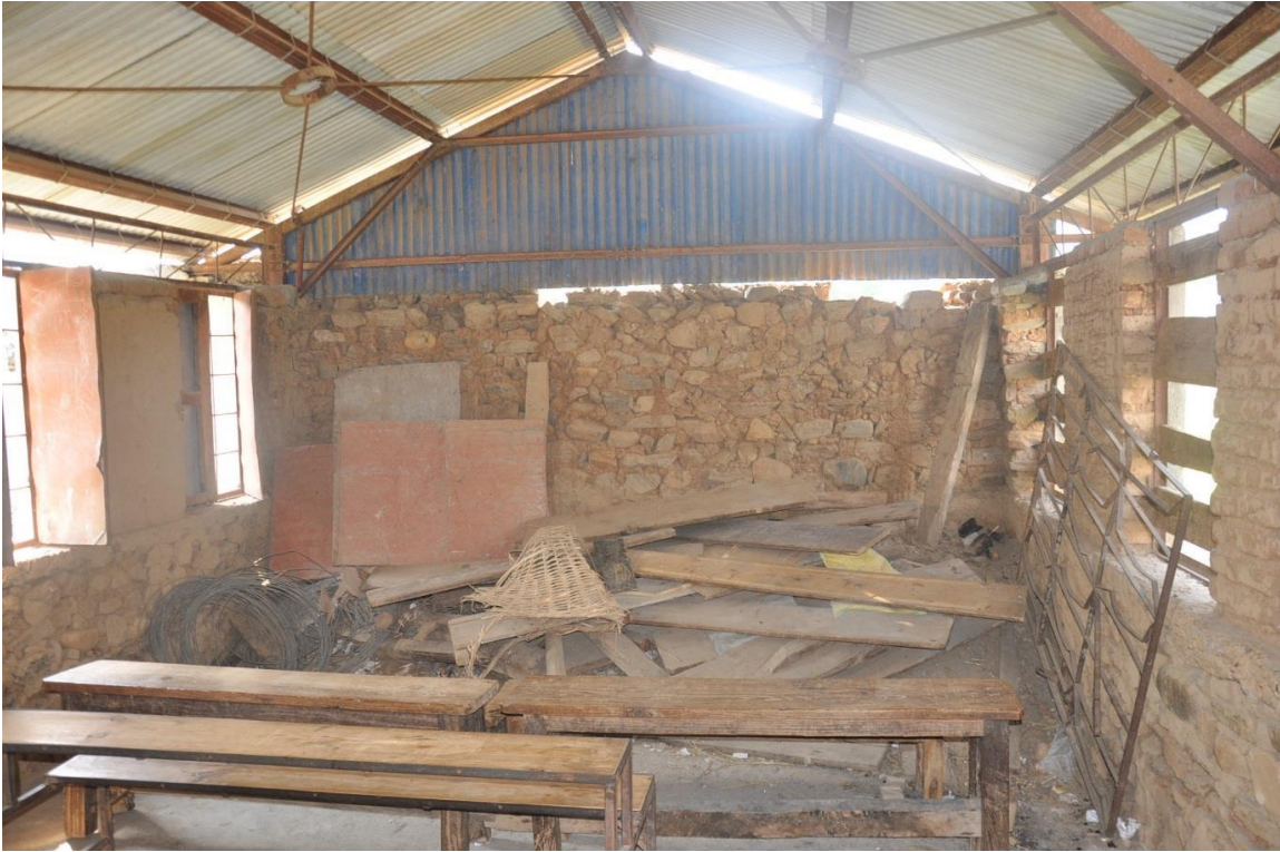
Earthquake damaged Classroom to be renovated.
