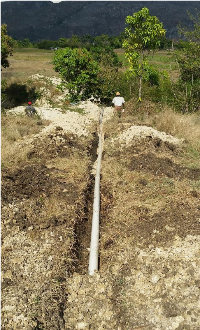
Gooding Rotary Project: Lines from pump to carry water to mango trees and additional acres
