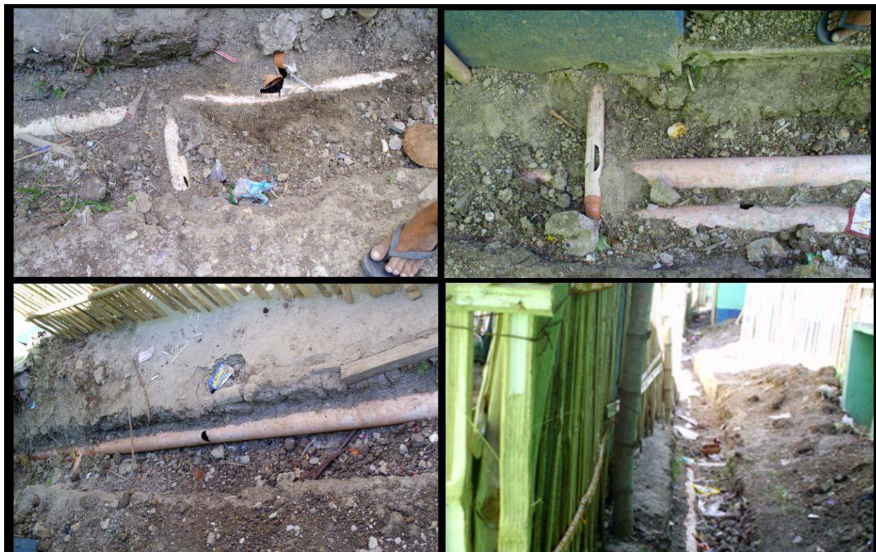
Picture No. 7: Damaged greywater lines.
