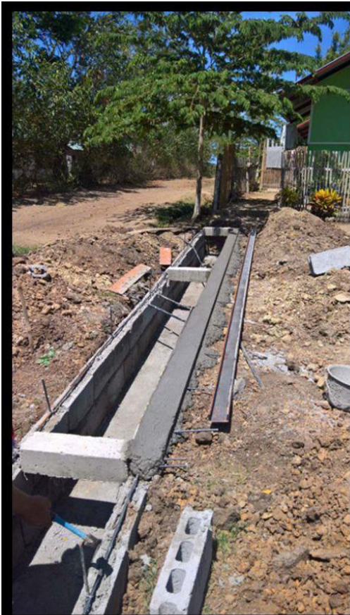
Phase 1: Canal terminated at the corner of the duplex unit at the upper right corner of the photo above.
