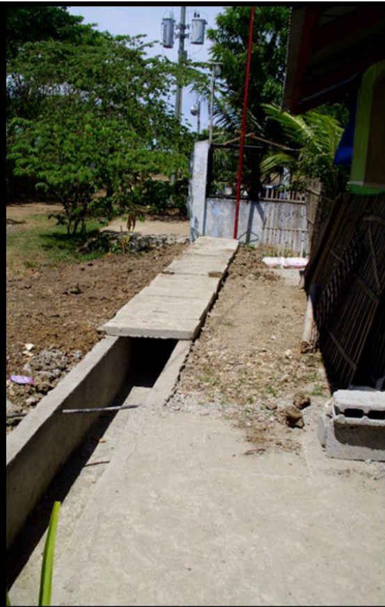
Phase 2: Canal terminated at the corner of the water utility's pumping station. Pre-cast concrete panels cover the portion in front of the duplex unit encroached upon by the project.
