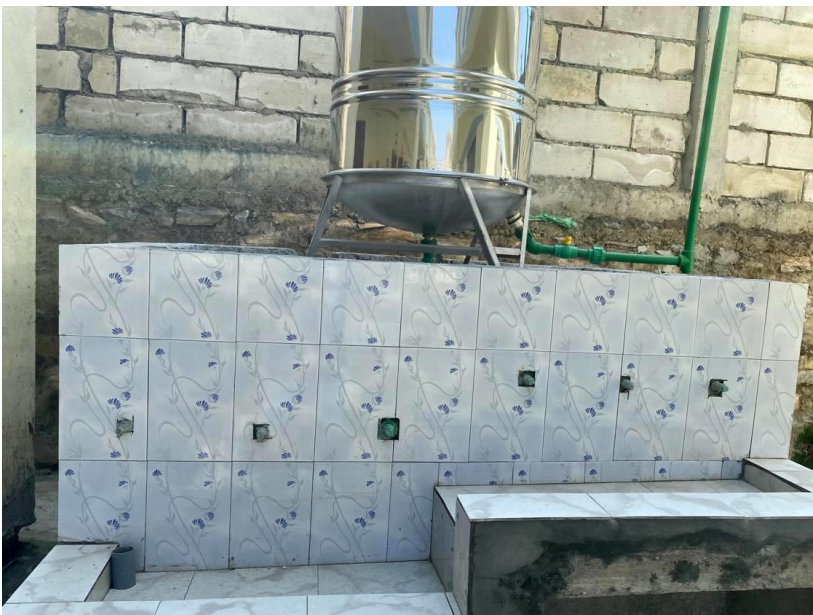
Completed new distribution facility with filtration system and water storage tank.
