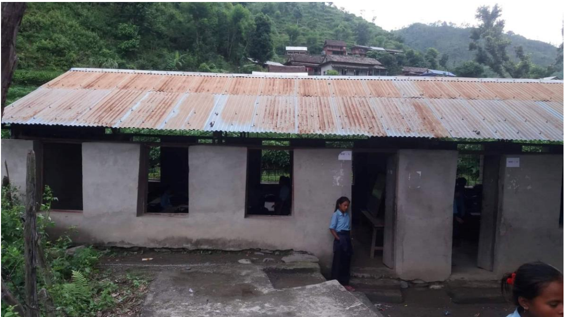
Front of Shree Bak School before repairs.
