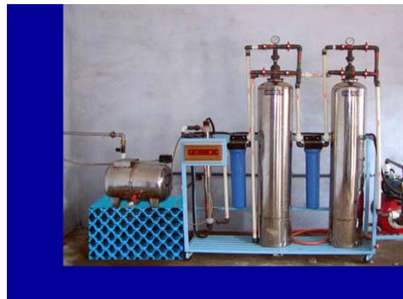
Filtration Plant Equipment
