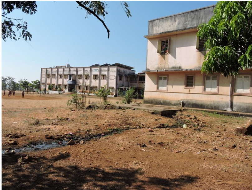
Free flowing overflow of septic tank
