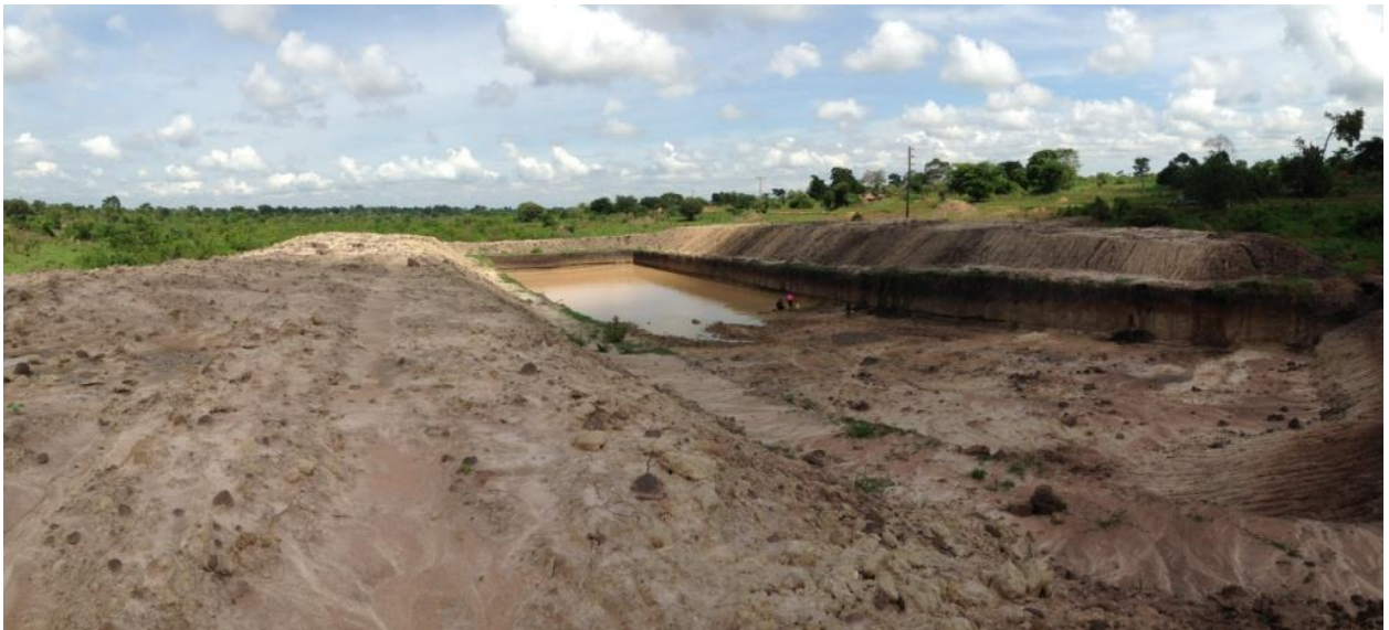
View of Kigeizere Valley tank showing need for final works.
