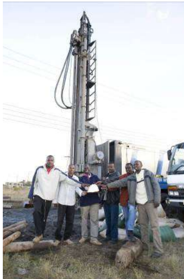
This is a Living Water Borehole Rig and the Crew. This photo represents Solution 1 to drill new boreholes.
