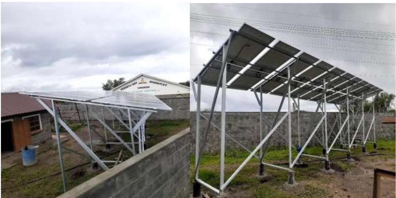
Ground Mount structure
