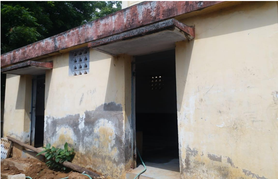
Pic 3: View of toilet Block building which is old, dilapidated and grossly inadequate
